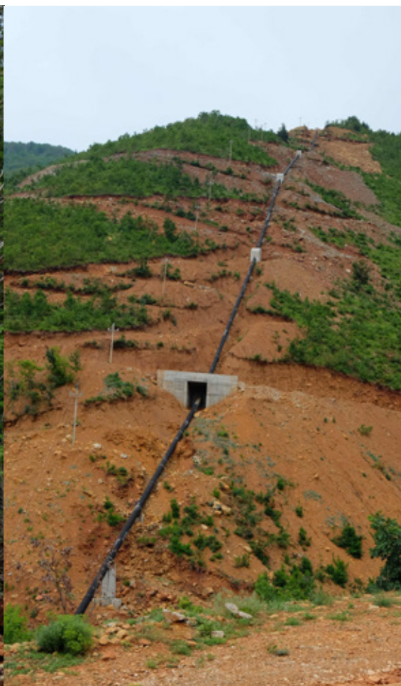
Figure 17: Erosion around the penstock
