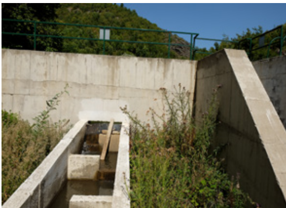
Figure 29: Blocked fish pass
