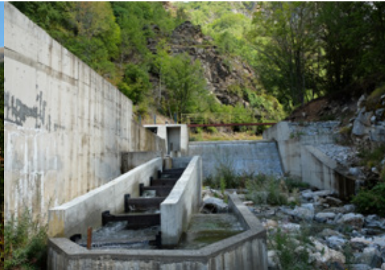
Figure 25: The intake with the new fish pass
