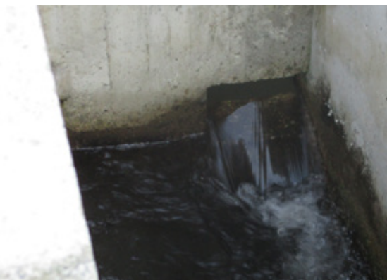
Figure 23: The upstream exit from the fish pass on Brajcinska intake
